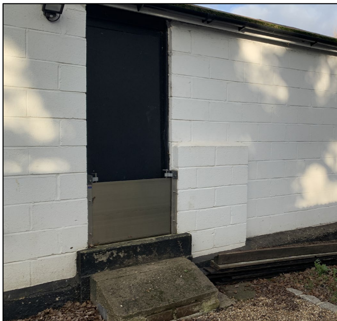
Flood barrier in place on a pavilion doorway ahead of a flood. Note that the door already has a raised threshold to help reduce flood ingress.
